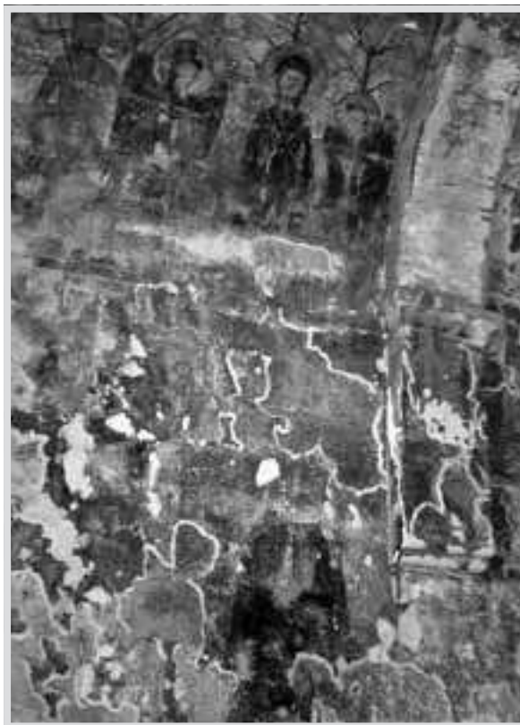
2 Different biodeterioration pattern in the western porch (left with respect to the entrance).
